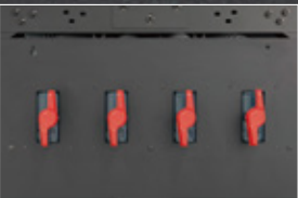
Vacuum zone valves
